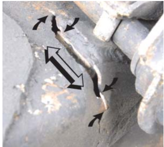
Figure 3. There's a lot of information in this photograph when you know how to interpret it. The two pairs of black arrows show the "new" crack propagation. The double headed arrow shows that portion of the crack that had previously fractured and propagated during service until it was well beyond the spacer pad. Note that the "old" fracture precisely follows the edge of the weld bead. That is typical. The ultimate cause of the dislocation shown was an accidental impact with a curb, but the structural failure was simply waiting to happen. The more these cracks propagate, the less energy it takes to open them up and cause a potential accident.
