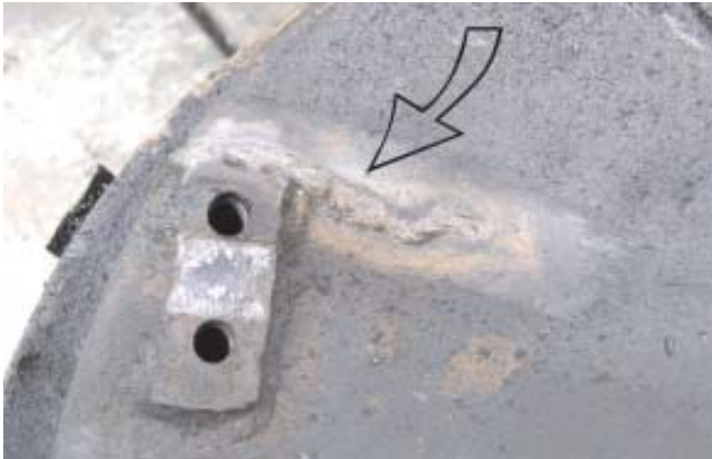
Figure 1. Here's a tell tale clue that this crossmember has seen previous repairs in its service life. The arrow shows the bead of weld that someone has placed over a former crack in the shell. You will also note in these photos that the entire perimeter of the spacer plates have been welded to the shell.
