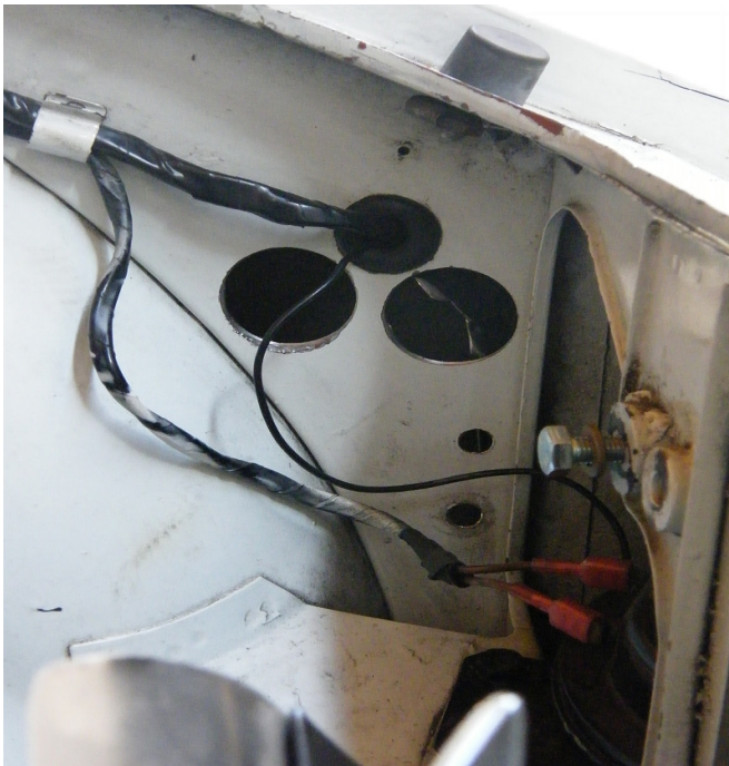
Figure 5 This is the side of the fender well after all the holes have been drilled. Now you can see why it's easier to hold the rubber bushings in place and mark the centers where you want the penetrations to go through the side. That way you can be sure that nothing gets in the way of having the hoses run through the bushings without overlapping or interference with other things in this area.
