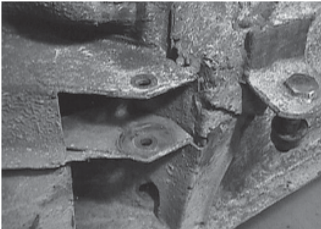
Figure 1. Inner Tie Plate Fracture
