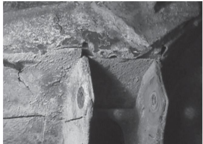
Figure 3. Crack in Triangular Gusset Plate
