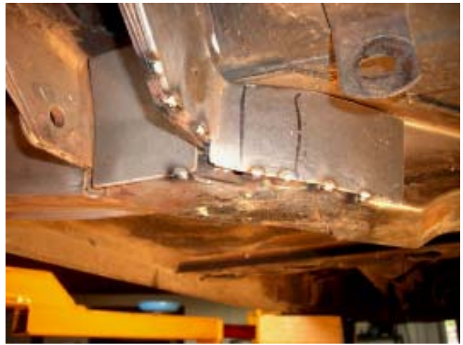
Figure 11. The first two pieces of reinforcement have been fit and tack welded into final position.
