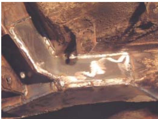
Figure 13. Here we have the finished application to the kit to the rear spring mount. Some minor weld dressing has been done and more can be done, but this gives you the general idea.
