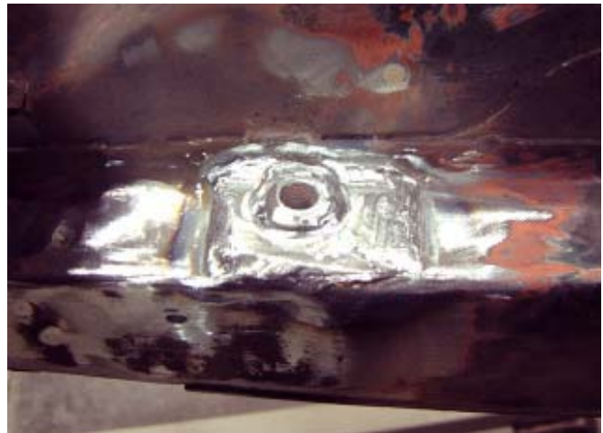
Figure 19. Here's the completed front tubenut reinforcement welded and completed. If you get this reinforcement piece applied before the tube nut starts its typical fatigue failure mode, you can save a lot of future problems and help keep your Tiger structurally sound.
