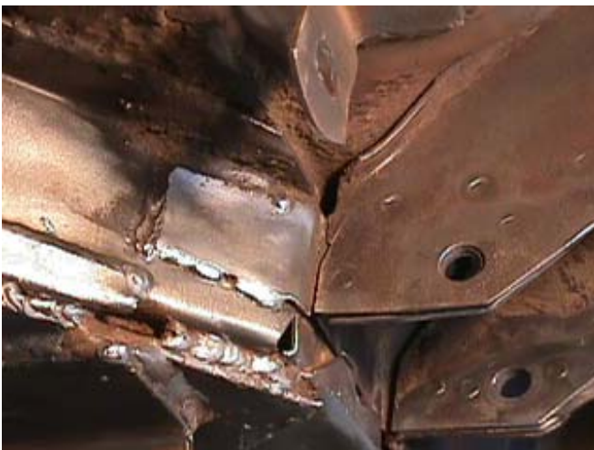
Figure 2. This is what most owners will find when they examine the front mounting area for the leaf springs. This crack is only the most visible failure point. It occurs because this location is a natural "hinge" in the chassis structure where the rear sub frame joins the body tub and X member.
