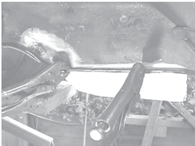
Figure 5. Here's the outer framerail clamped back in position with vise grips. This entire length should be welded, from the arch forward to the end of the three layer lamination. You can simply fuse the edges together or drill holes and plug weld this flange. Be sure to grind any weld bead that protrudes below the flat surface.
